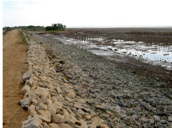
Figure 4-6: In places with high erosion, natural regeneration is not possible; mangrove forests are destroyed and waves affect the dyke
