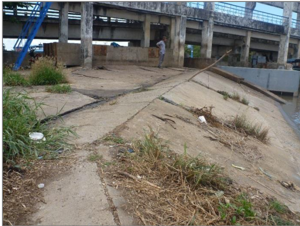
Figure 3-15 Settling of concrete plates, sluice 10 (Sikora)
