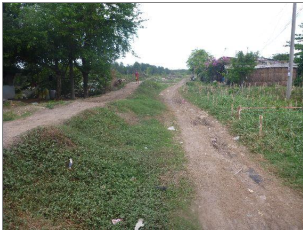
Figure 3-8 Difference in height at the dike surface at km (-41) (Sikora)
