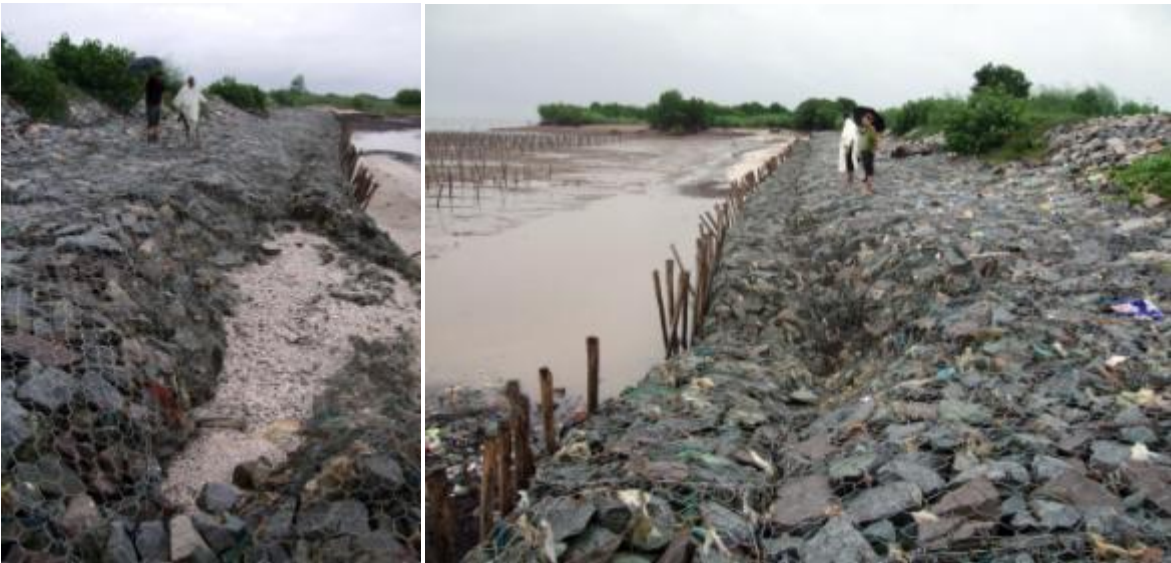
Failure of the outer slope of the endangered dyke at Vinh Tan in October 2010; Photo GIZ
