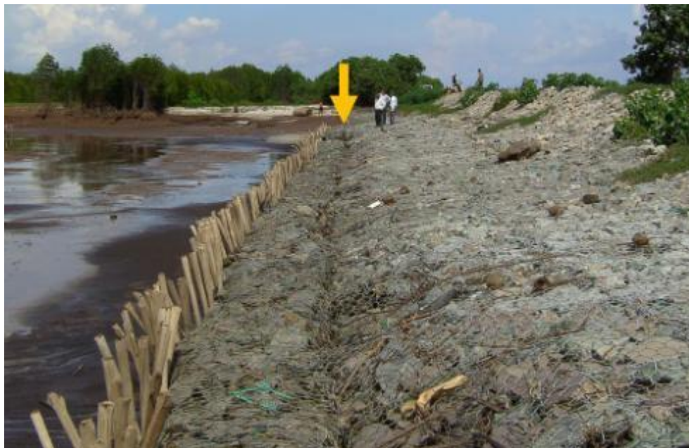
Figure 5: Photo of the improved dyke at Vinh Tan with a gap in the revetment due to further erosion.
