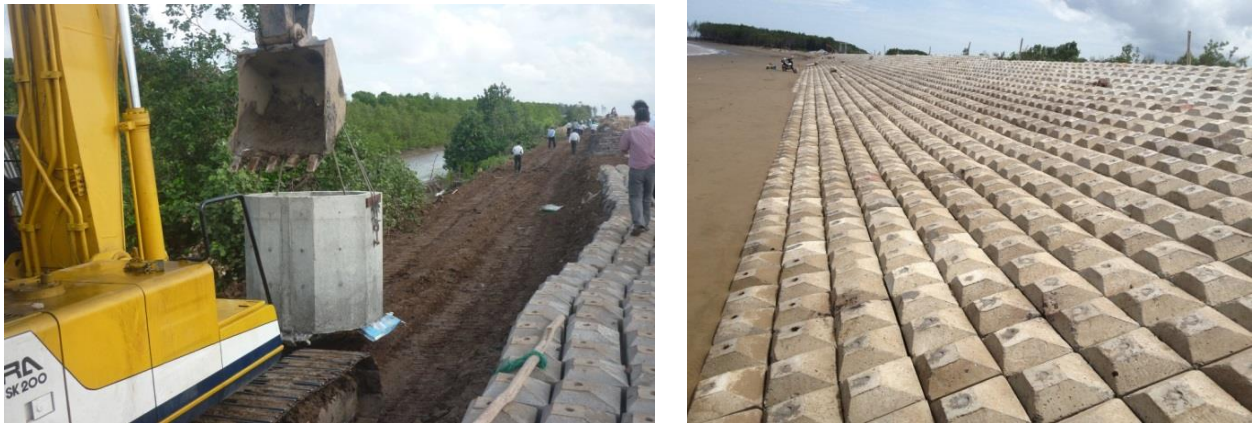
Figure 5a-c: Dike revetments and mangrove plantation in Soc Trang (Province of Soc Trang)
