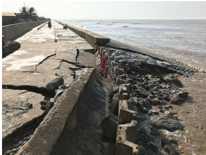
Figure 4: Severely damaged revetment in Ganh Hao (Source: Province of Bac Lieu)
