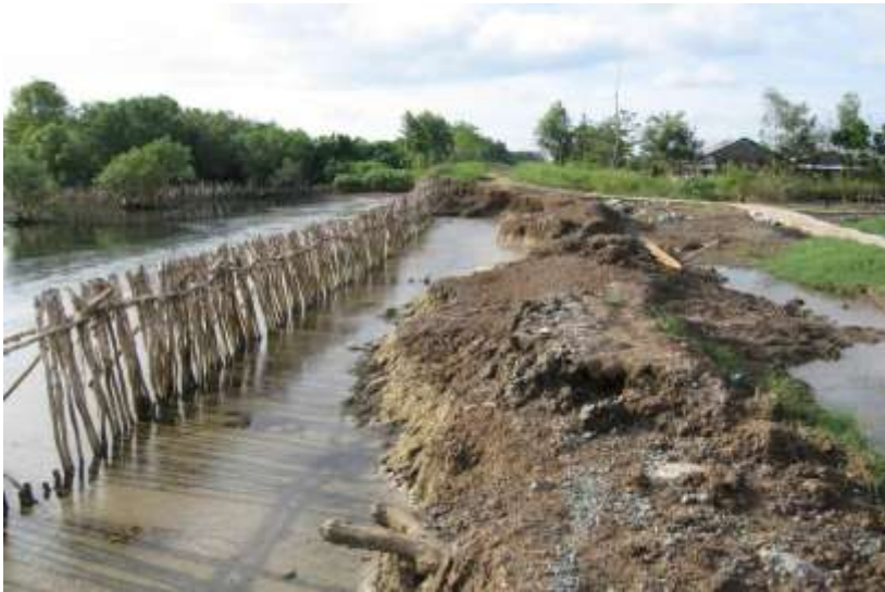
Photo 19: in-homogenous dam material
