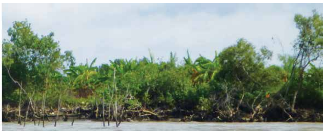
Active erosion; there is a high erosion scarp and most of the fringing mangroves have been eroded, exposing the terrestrial vegetation and crops (bananas) in the hind shore.
