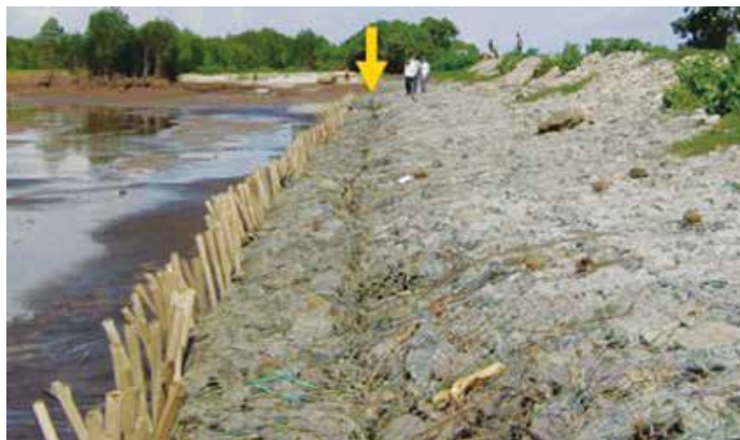
Figure 4: Toe protection with wood piling. Yellow arrow: Gap in revetment due to further erosion [Albers & Von Lieberman, 2011]
