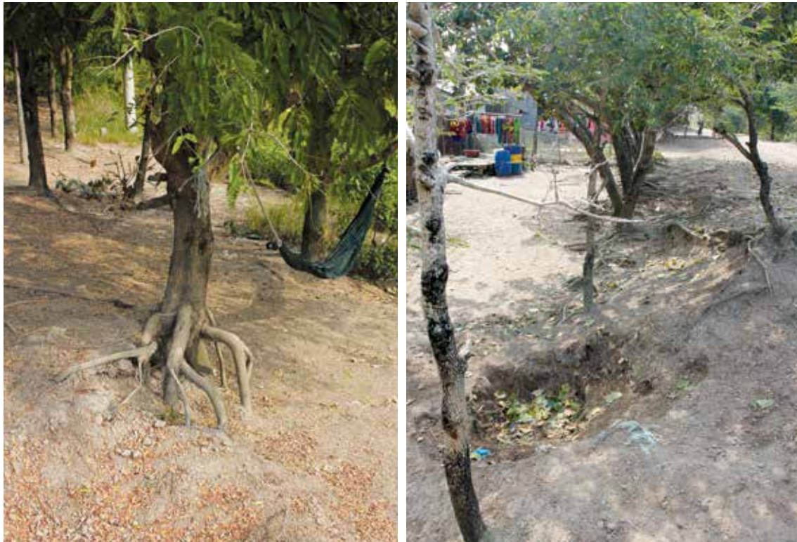
Figure 20: Tree on dike slope with exposed roots (left) and break out on dike slope (right)
