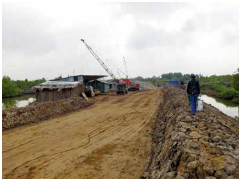
Figure 14: Dike construction works nearby the bridge to build a road on the dike
