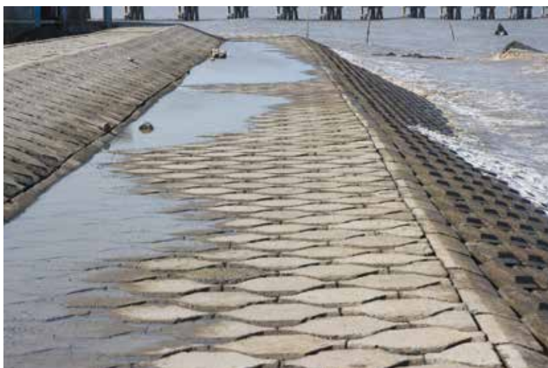
Figure 26: Settlements of the seaward berm filled with standing water
