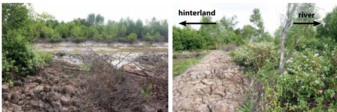
Figure 13: View from the dike crest towards the channel Song Cua Lon (left) and view along the dike line (right) (03.01.2014 #4)
