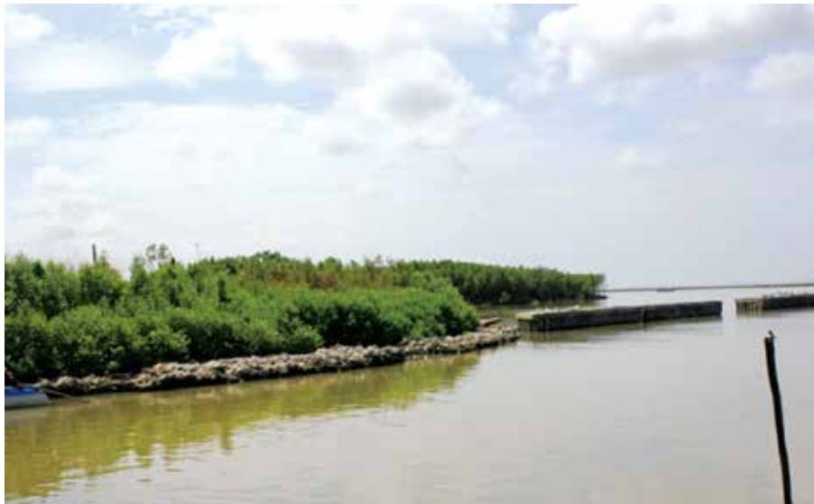
Figure 37: Gabion protection at sluice gate in Khanh Tien/ Khanh Hoi commune and connected breakwater
