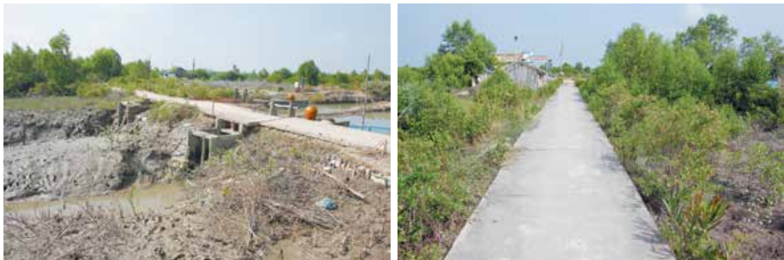
Figure 18: Embankment with road in front of the milestone line next to the channel
