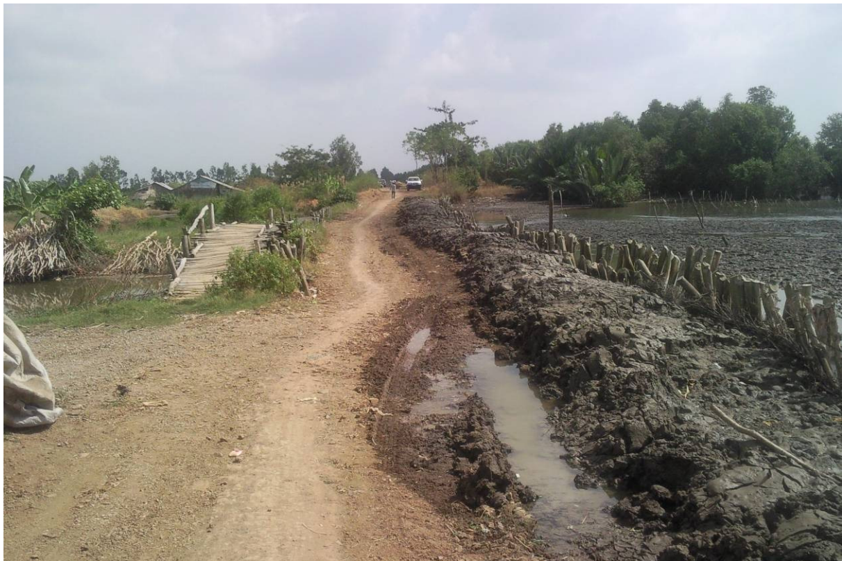
Fig.6: Eroded dyke with emergency repair in Hon Dat district
