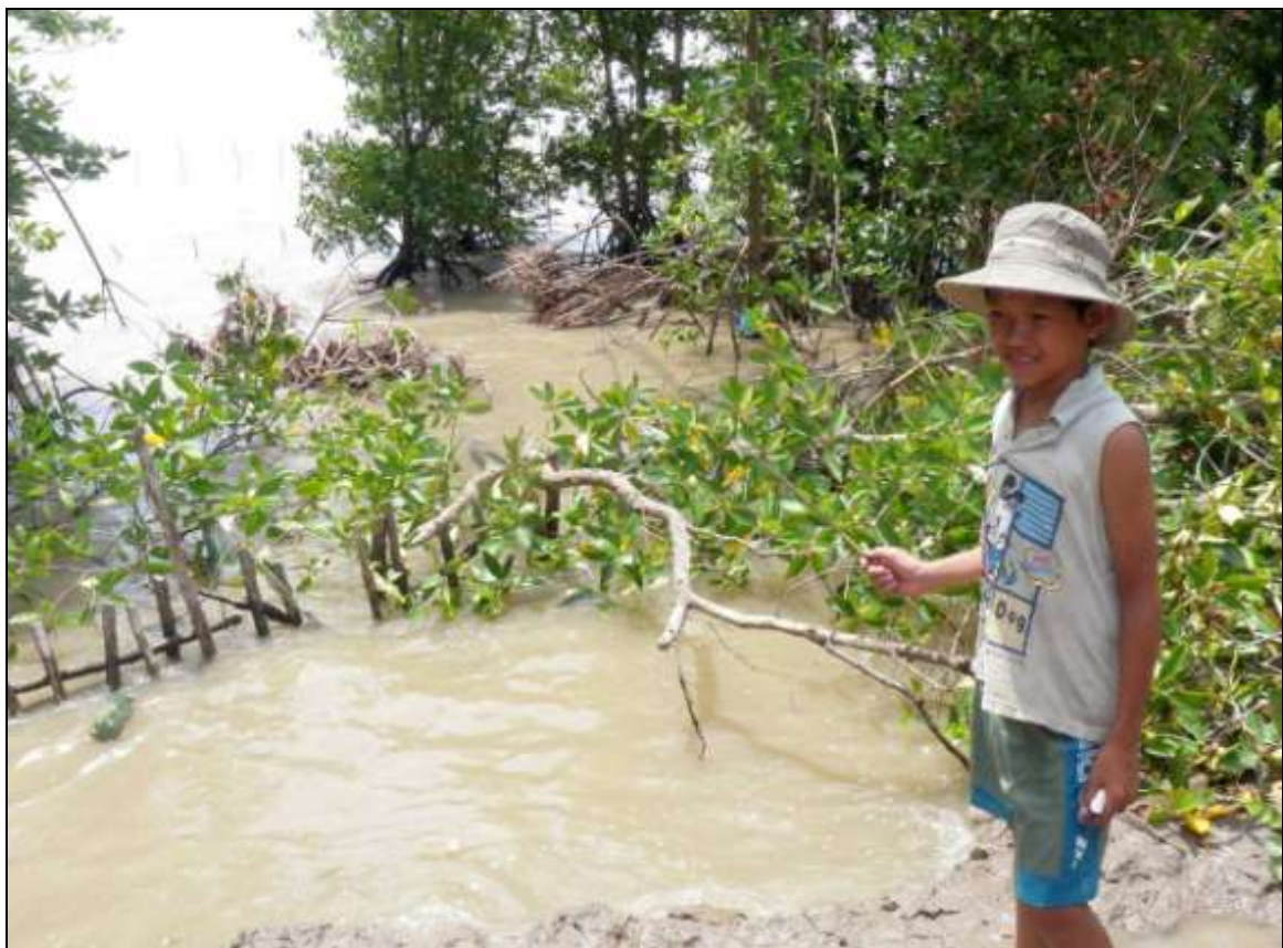
Figure 9: Sea broken through the thin remaining mangrove fringe, threatening the small dyke enclosing aquaculture pond, An Bien.
