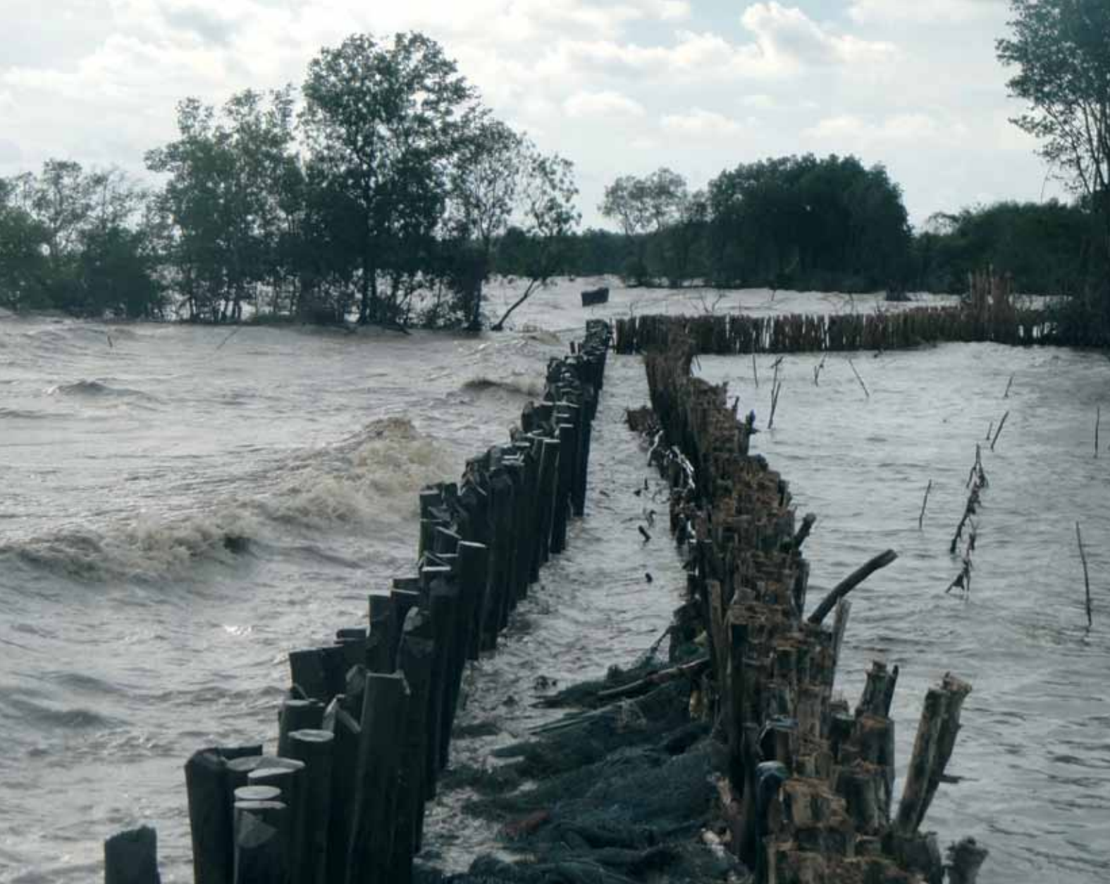
Wave break fence for high erosion areas.
