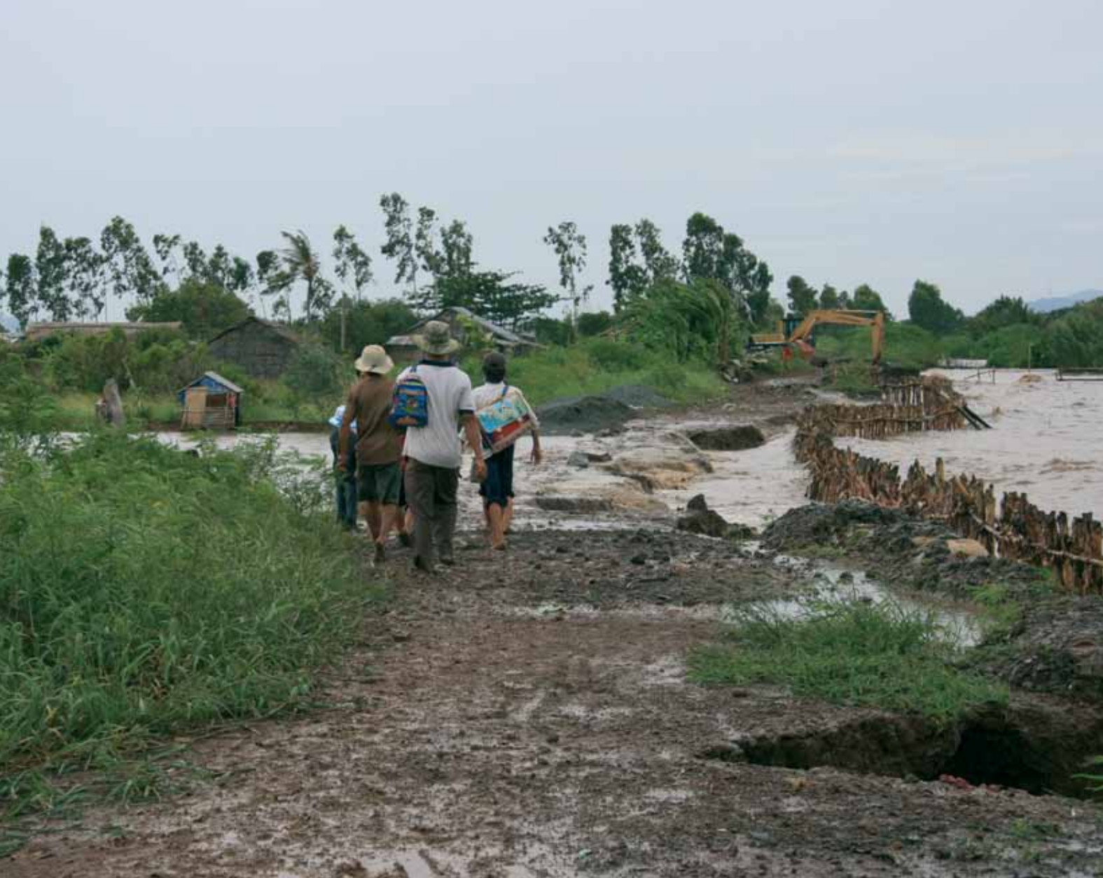
Protection earthen dykes were breached annually before work started in the Vam Ray demonstration area.
